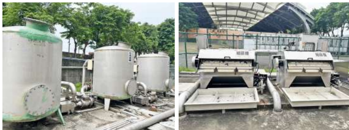
▲ Sewage treatment plant at the Yanchao Campus
