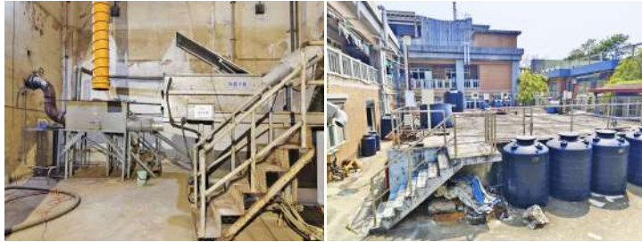
▲ Photo of Sewage treatment plant at the First Campus
