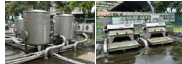
▲ Sewage treatment plant at the Yanchao Campus
