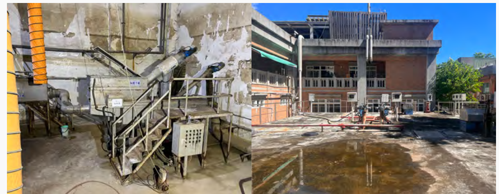
▲ Sewage treatment plant at the First Campus
