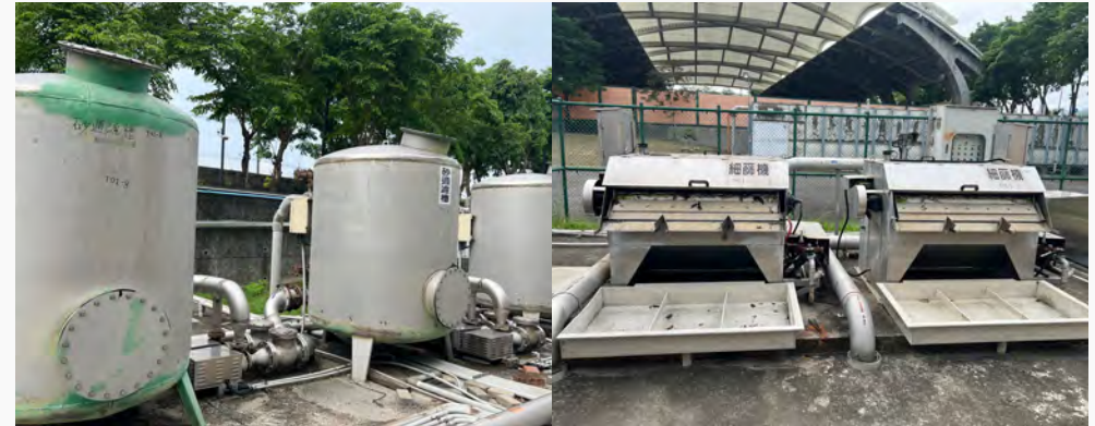
▲ Sewage treatment plant at the Yanchao Campus
